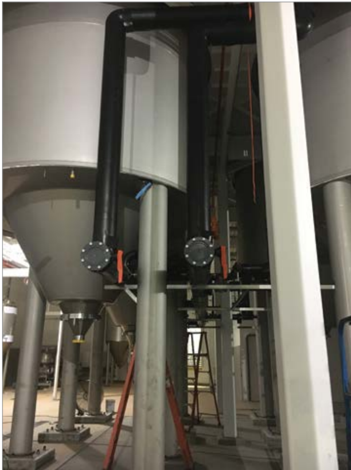
Shown is one of 16 new 60-foot tanks in the Bay 7 Loop Project. The expansion included a run of 1,000 feet of COOL-FIT piping to convey chilled water to keep the beer tanks cold.
