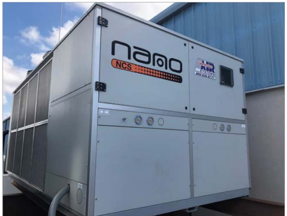
Compressed Air Systems installed the nano model NCS-1004-US 43-ton, water-cooled, cycling chiller on the roof of Coppertail's microbrewery.
